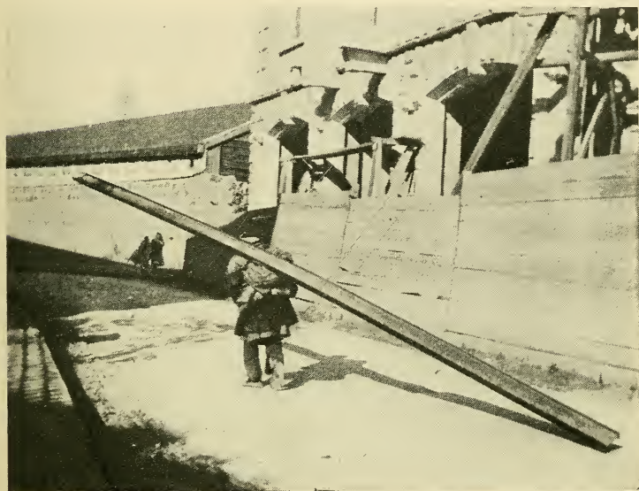
The Palestine beast of burden carrying an iron beam to a building in construction
